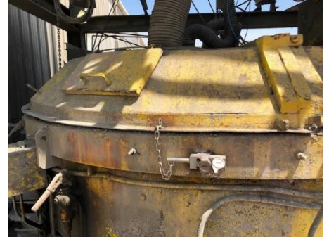
KIRK Type DM installed on mixer – it is now safe to access mixer and perform maintenance.
