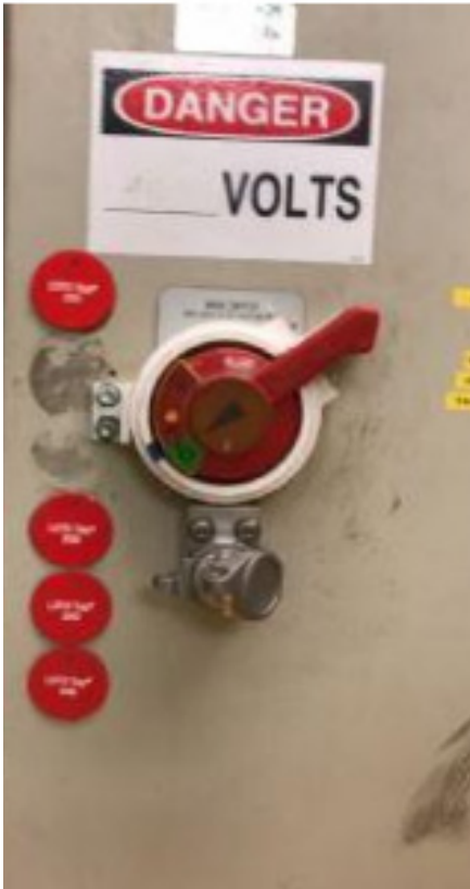
KIRK Applied Engineering Services custom collar solution, installed on customer's equipment, with Type F interlock for power isolation.
