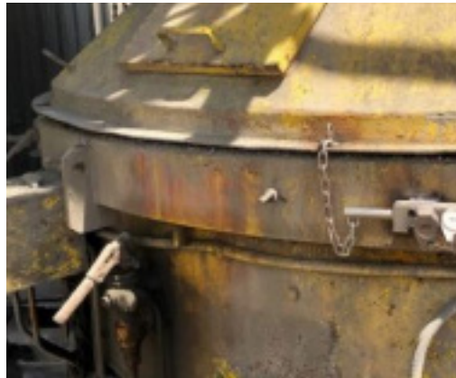
KIRK Type DM installed on mixer – it is now safe to access mixer and perform maintenance.
